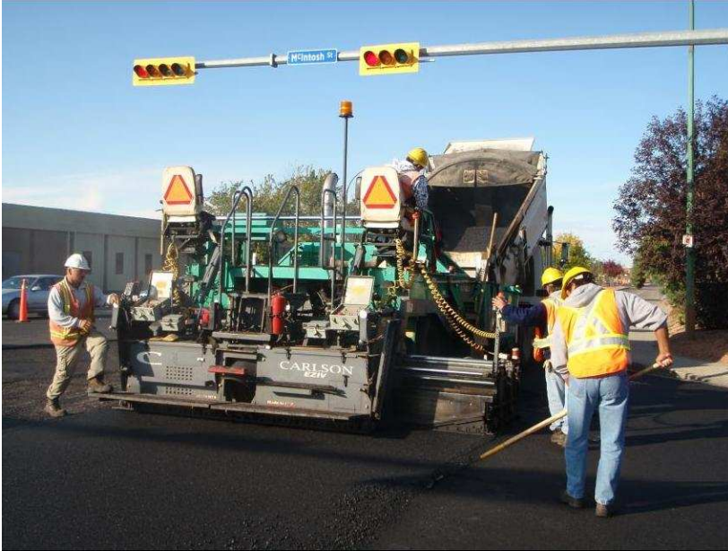
City Crews Milling and Paving as part of Street Infrastructure Renewal Program
