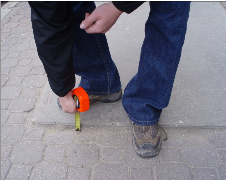
Measurement of Vertical Displacement (Step) on Sidewalk
