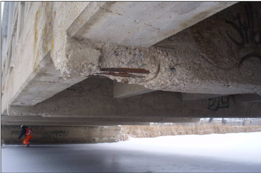
View of Bridge Structure with Exposed Steel Bars
