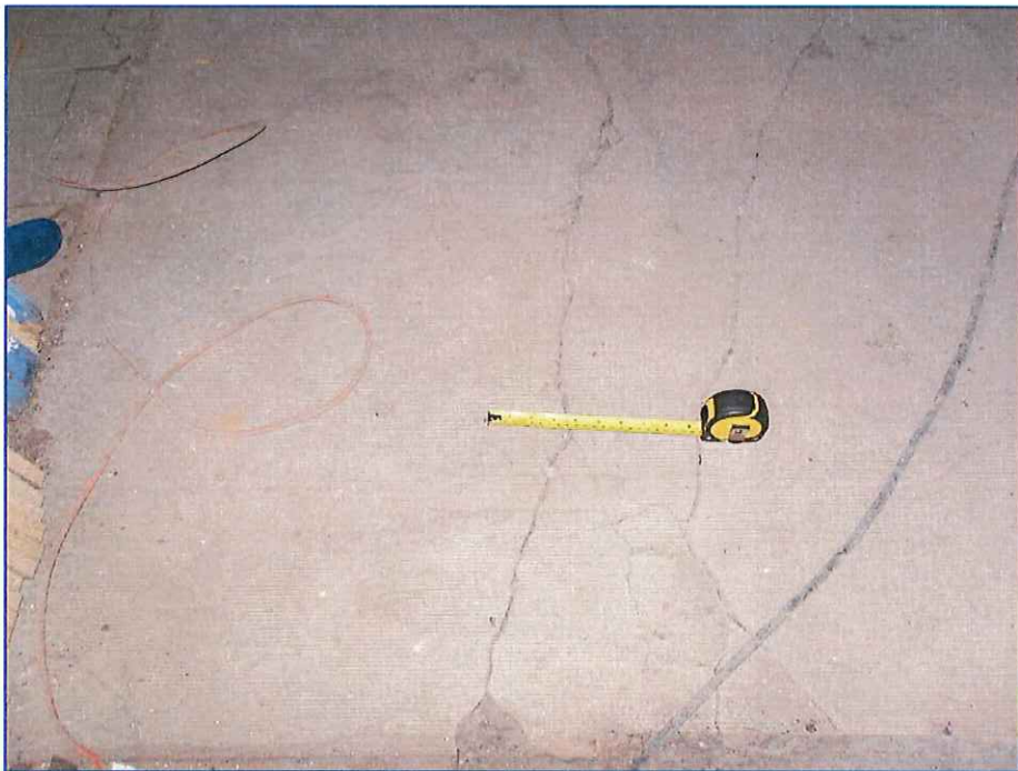
Photo 6 – Heaving and Cracking in Main Floor Slab on Grade
