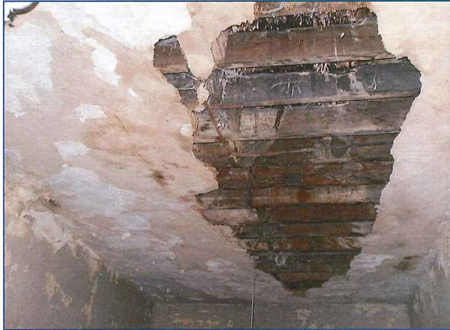
Photo 13 – Exposed Roof Joists (Water Discoloration Evident)
