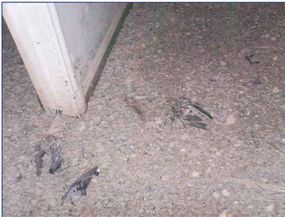
Photo 12 – Bird Feces and Bird Remains on Second Floor
