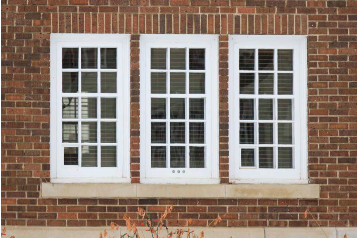
Caption: Detail of a triple assembly window with wood sashes, storms, with brick mullions and lintel, on the front elevation of the Willoughby Residence.
