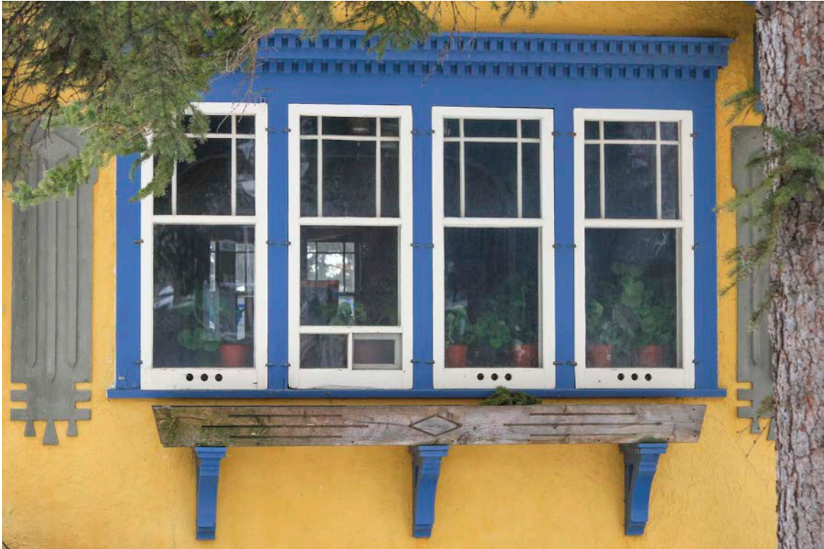
Caption: Detail of the wood window assembly on the front elevation of the Cassidy Residence.
