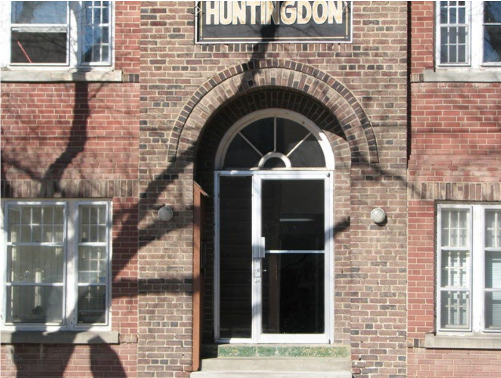
Recessed front entry arched transom and curved brick lintel, 2010 (City of Regina)
