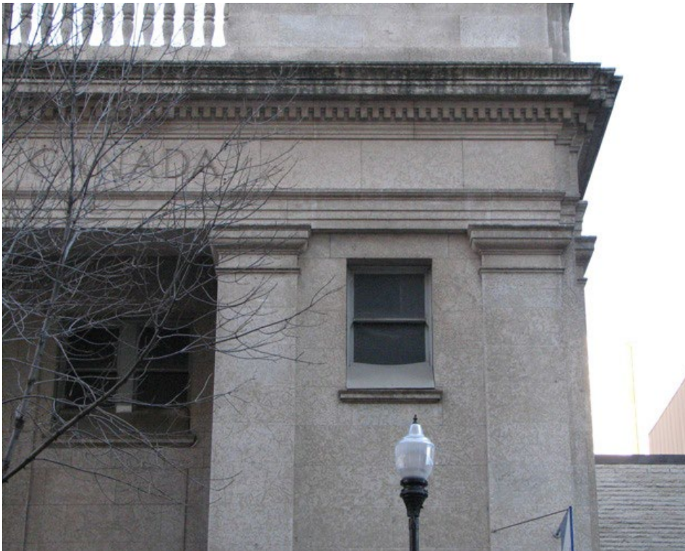
Detail of the engaged Tyndal stone square columns, frieze, and cornice on the south elevation of the Merchants Bank of Canada, 2010 (City of Regina)
