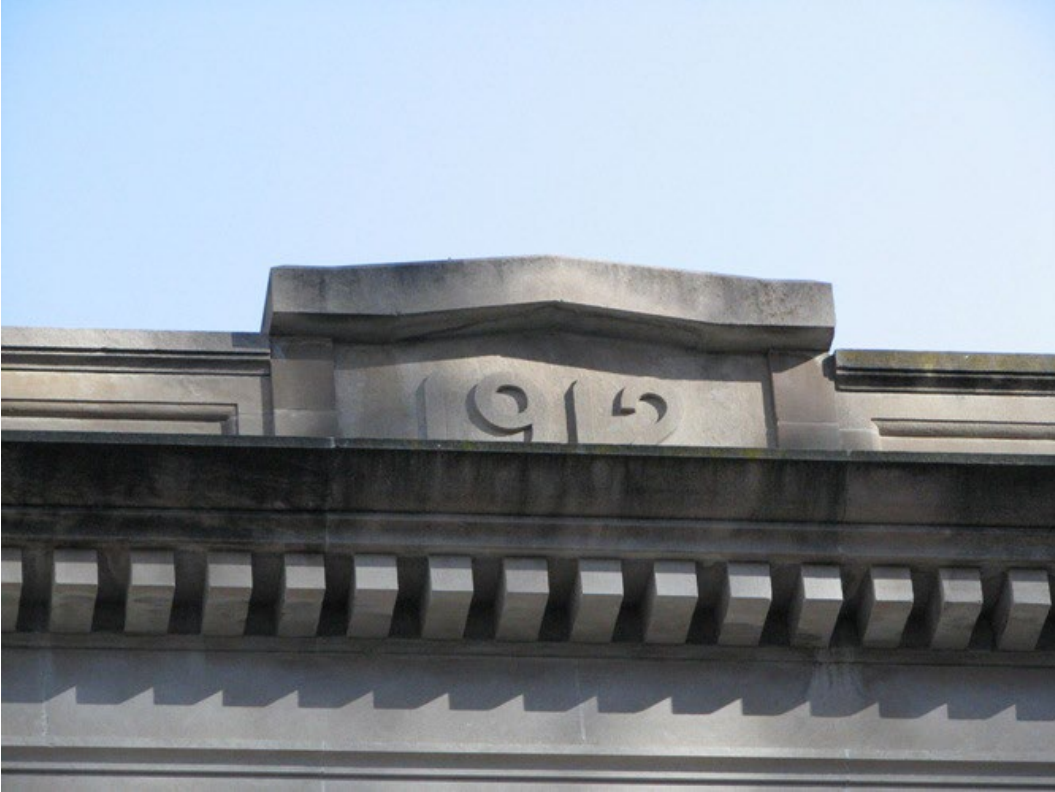
Stone parapet with date of construction crest and stone cornice with dentils, 2010 (City of Regina).
